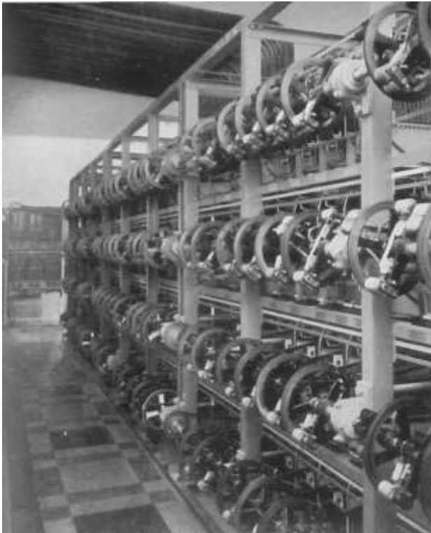
Left. Multiple dimmer bank relays operated from the Strand Light Console, National Opera House, Lisbon (1940) Note vi .
